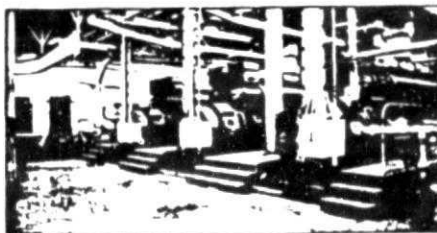
Three EMD Diesel Engine Generator Sets.
